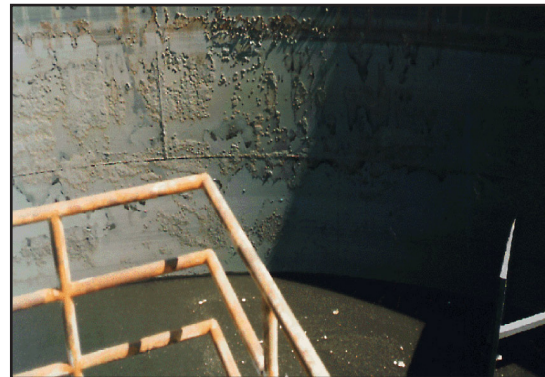
Failed coal tar epoxy coating
